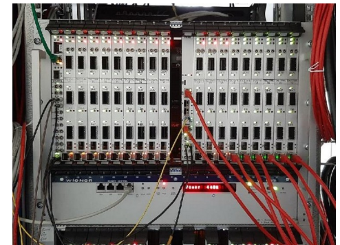
VME-VXS crate with TDC modules, trigger and synchronization module.
